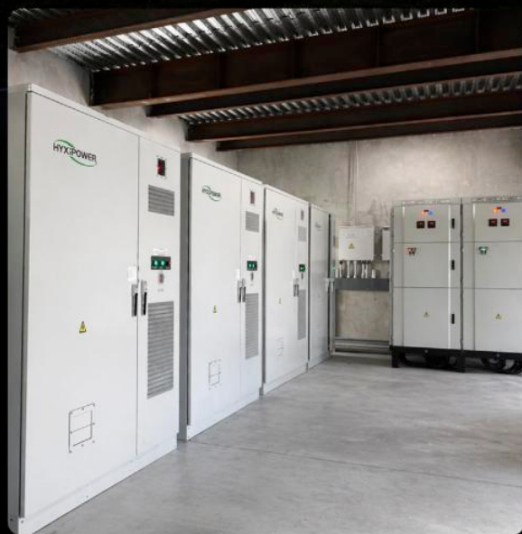
105kW/232kWh C&I ESS Myanmar, Capacity 500kW/1075kWh
