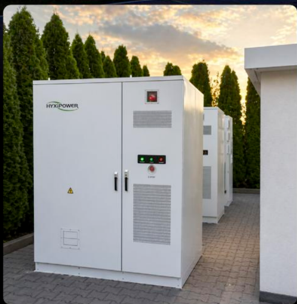
100kW/215kWh C&I ESS Poland, Capacity 200kW/430kWh
