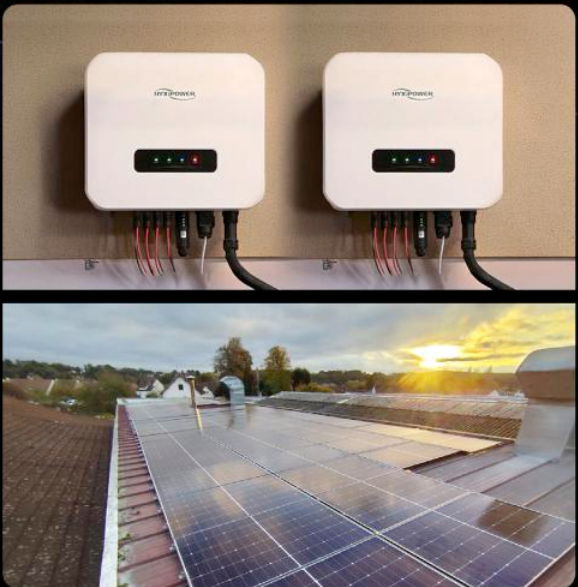
String Inverter Eure-et-Loir, France, Capacity 45kW
