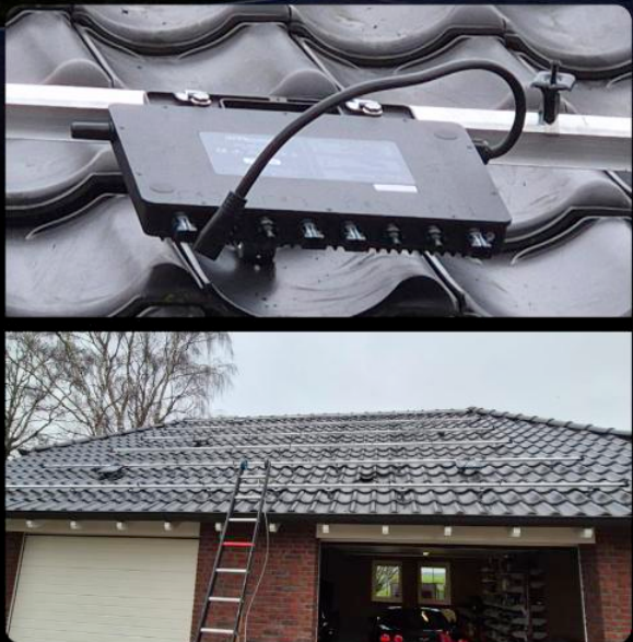
Microinverter Drenthe, Netherlands, Capacity 7.9kW
