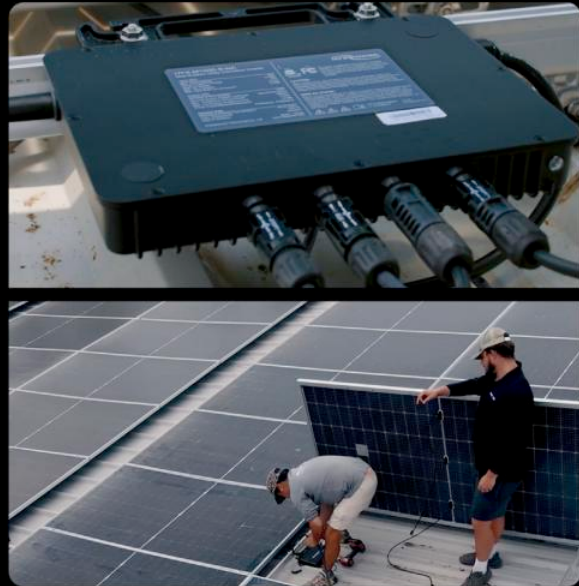
Microinverter Texas, USA Capacity 117kW
