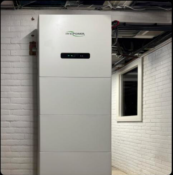
All-in-One ESS Overijssel, Netherlands, Capacity 12kW/20kWh
