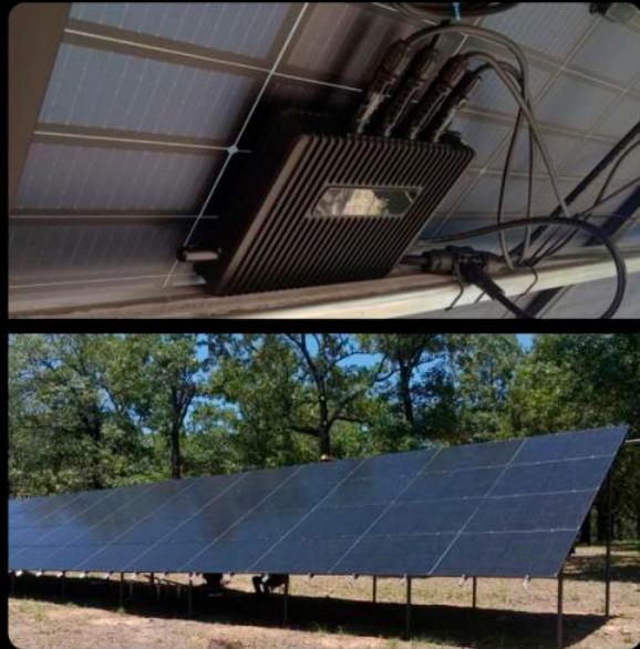
Microinverter Arkansas, USA, Capacity 11.6kW
