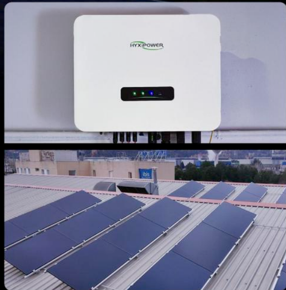
Hybrid Interter Barcelona, Spain, Capacity 25kW
