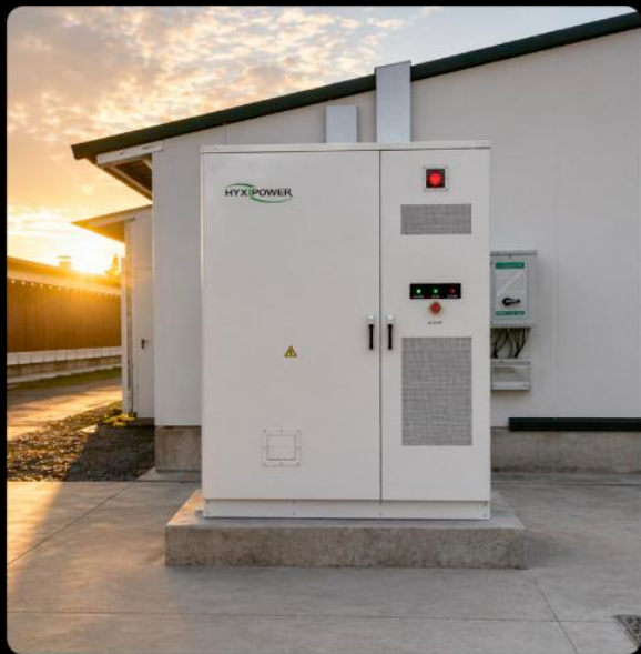
105kW/232kWh C&I ESS Spain, Capacity 100kW/215kWh
