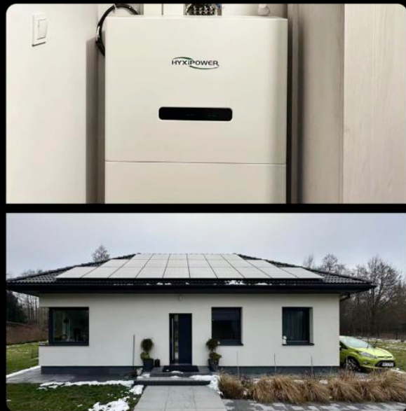
All-in-One ESS Mazovia, Poland, Capacity 10kW
