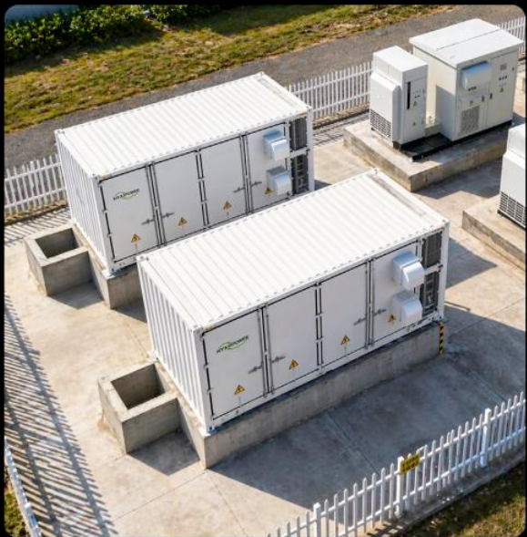
5000kWh Container ESS Zhejiang, China, Capacity 5MW/10MWh
