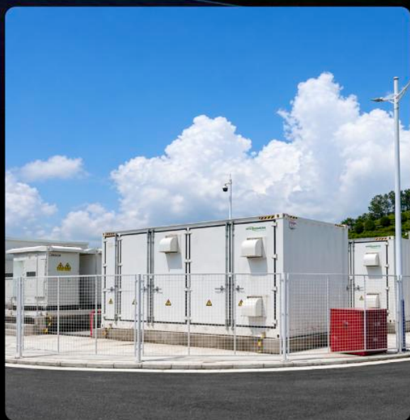
5000kWh Container ESS Zhejiang, China, Capacity 400MWh
