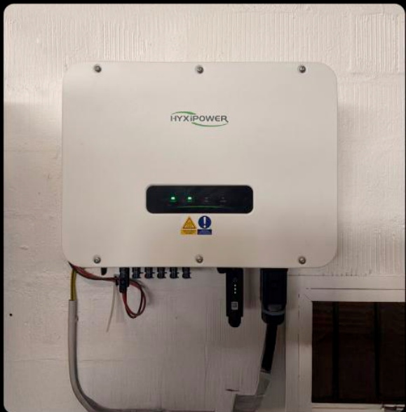
Microinverter Drenthe, Netherlands, Capacity 7.9kW
