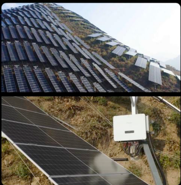
String Inverter Hangzhou, China, Capacity 40MWp
