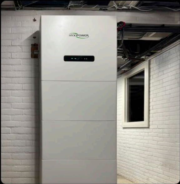
All-in-One ESS Overijssel, Netherlands, Capacity 12kW/20kWh
