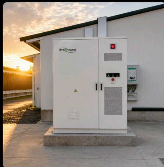
105kW/232kWh C&I ESS Spain, Capacity 100kW/215kWh
