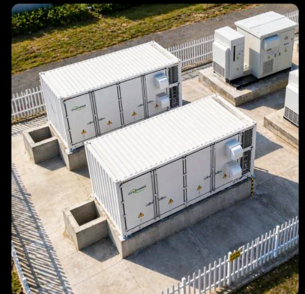
5000kWh Container ESS Zhejiang, China, Capacity 5MW/10MWh
