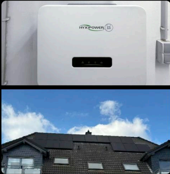
Hybrid Inverter & High Voltage Battery Rheinland-Pfalz, Germany, Capacity 50kW
