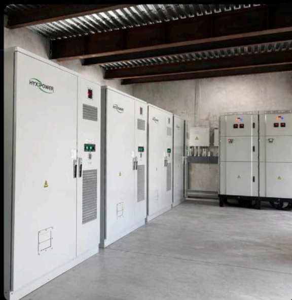
105kW/232kWh C&I ESS Myanmar, Capacity 500kW/1075kWh
