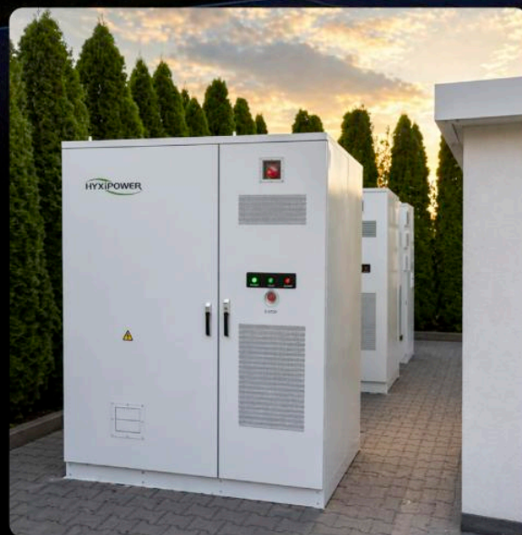
100kW/215kWh C&I ESS Poland, Capacity 200kW/430kWh
