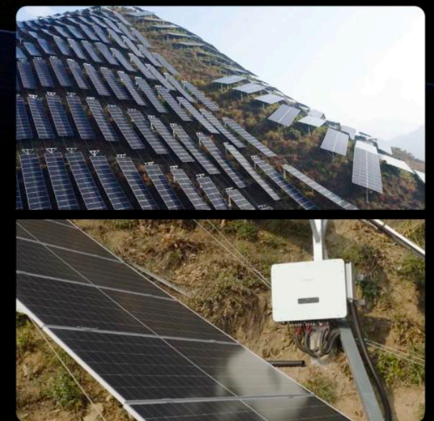
String Inverter Hangzhou, China, Capacity 40MWp
