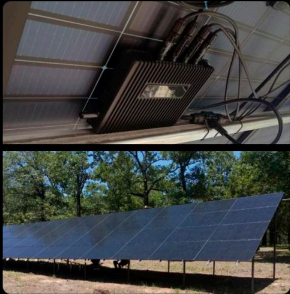
Microinverter Arkansas, USA, Capacity 11.6kW
