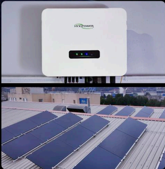
Hybrid Interter Barcelona, Spain, Capacity 25kW
