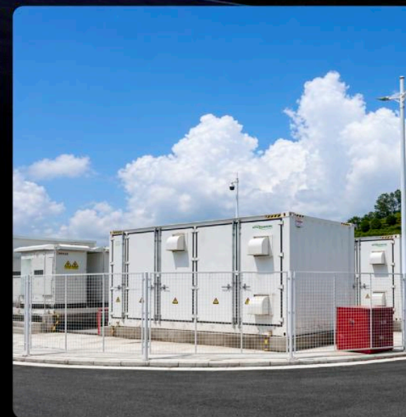
5000kWh Container ESS Zhejiang, China, Capacity 400MWh
