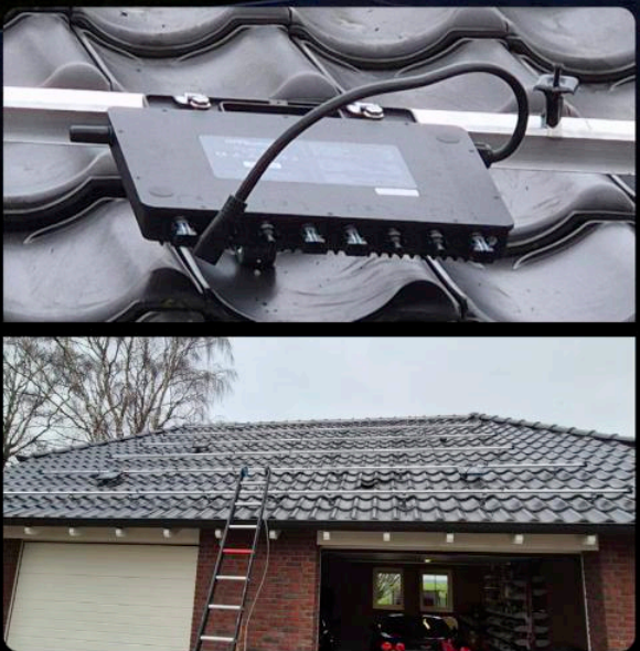
Microinverter Drenthe, Netherlands, Capacity 7.9kW
