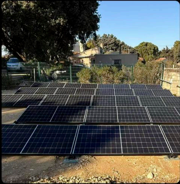
Microinverter Orange, France, Capacity 9kW
