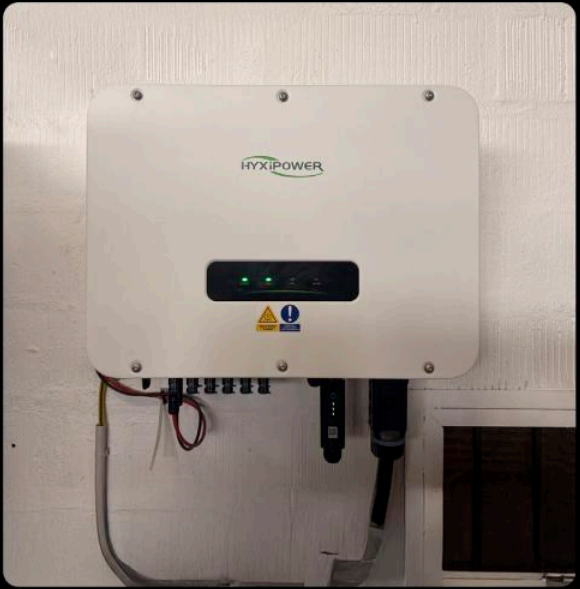
Microinverter Drenthe, Netherlands, Capacity 7.9kW
