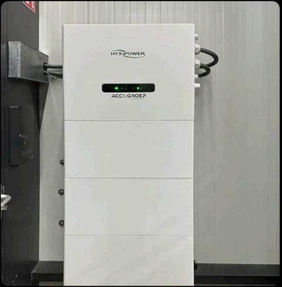
All-in-One ESS Overijssel, Netherlands, Capacity 12kW/20kWh
