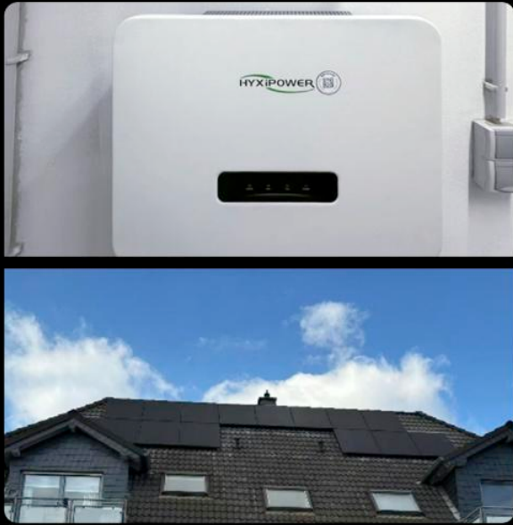
Hybrid Inverter & High Voltage Battery Rheinland-Pfalz, Germany, Capacidade 50kW
