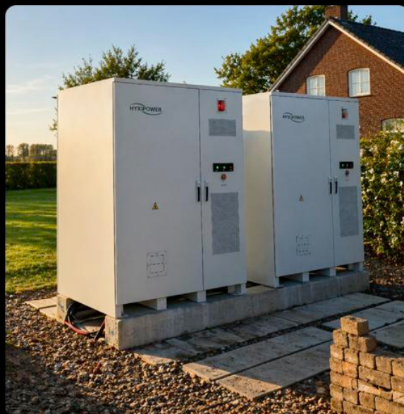
105kW/232kWh C&I ESS Netherlands, Capacidade 200kW/430kWh
