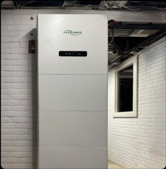
All-in-One ESS Overijssel, Netherlands, Capacity 12kW/20kWh
