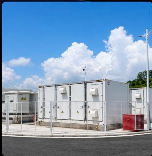
5000kWh Container ESS Zhejiang, China, Capacity 400MWh
