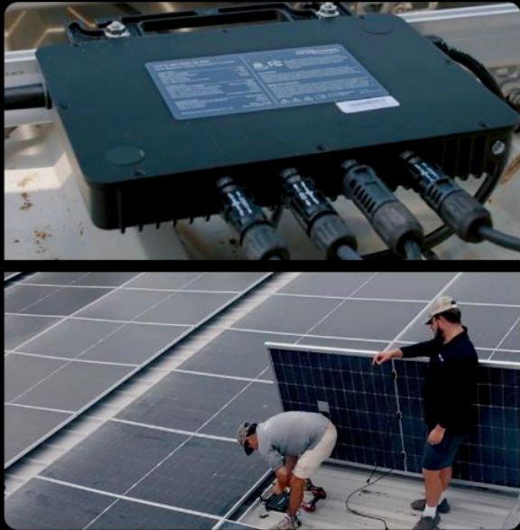
Microinverter Texas, USA Capacity 117kW
