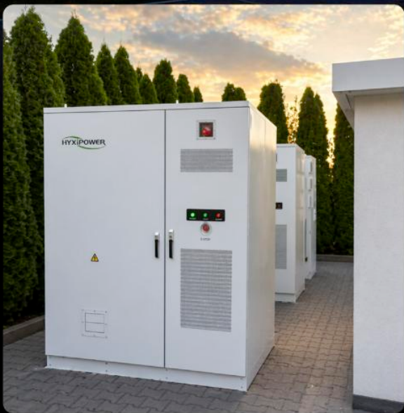
100kW/215kWh C&I ESS Poland, Capacity 200kW/430kWh
