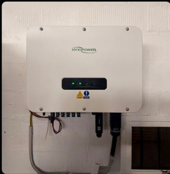
Microinverter Drenthe, Netherlands, Capacity 7.9kW
