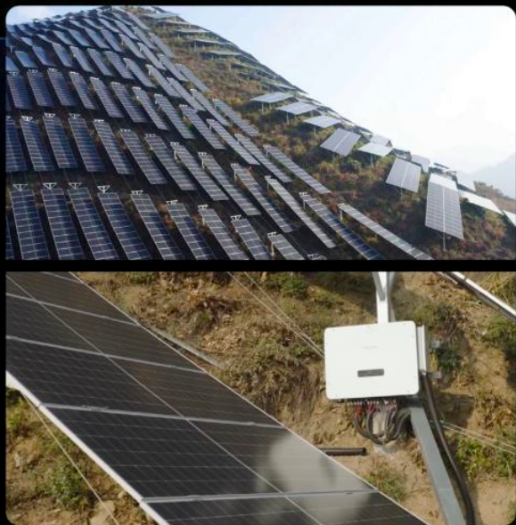
String Inverter Hangzhou, China, Capacity 40MWp
