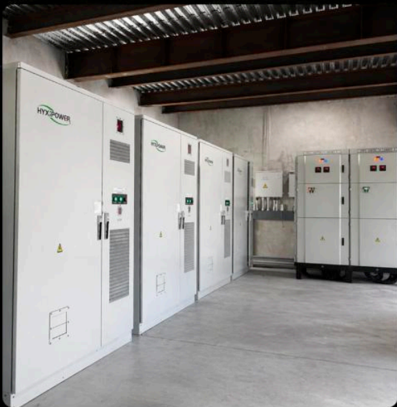
105kW/232kWh C&I ESS Myanmar, Capacity 500kW/1075kWh
