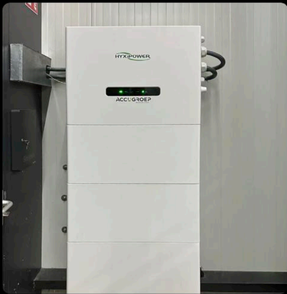
All-in-One ESS Overijssel, Netherlands, Capacity 12kW/20kWh
