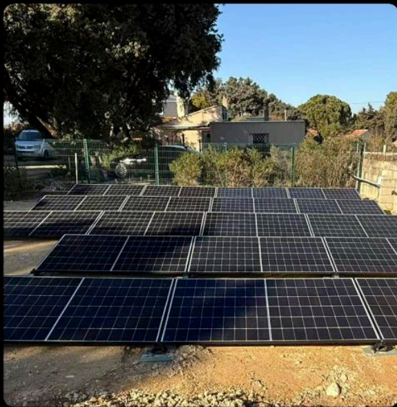
Microinverter Orange, France, Capacity 9kW
