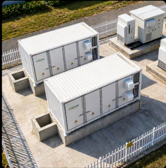
5000kWh Container ESS Zhejiang, China, Capacity 5MW/10MWh
