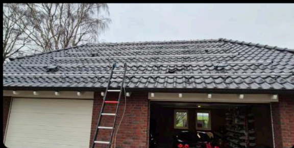
Microinverter Drenthe, Netherlands, Capacity 7.9kW
