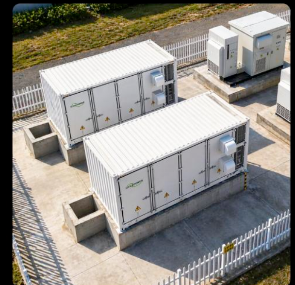
5000kWh Container ESS Zhejiang, China, Capacity 5MW/10MWh
