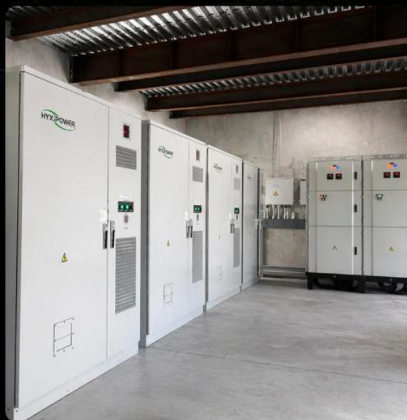
105kW/232kWh C&I ESS Myanmar, Capacity 500kW/1075kWh
