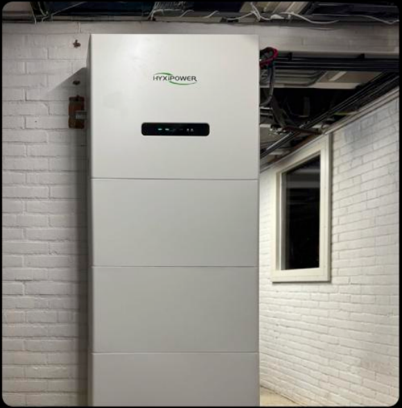
All-in-One ESS Overijssel, Netherlands, Capacity 12kW/20kWh
