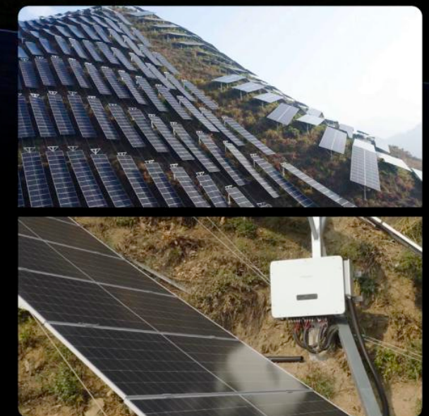
String Inverter Hangzhou, China, Capacity 40MWp
