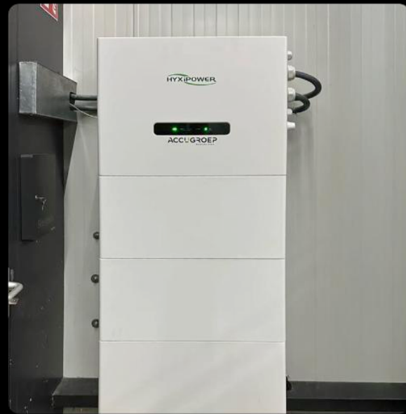
All-in-One ESS Overijssel, Netherlands, Capacity 12kW/20kWh
