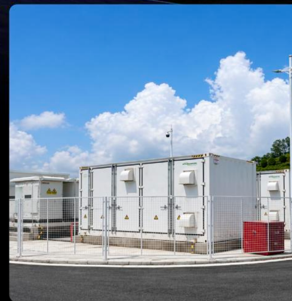
5000kWh Container ESS Zhejiang, China, Capacity 400MWh
