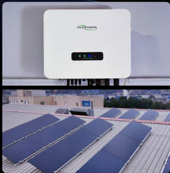
Hybrid Interter Barcelona, Spain, Capacity 25kW
