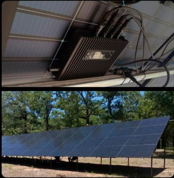
Microinverter Arkansas, USA, Capacity 11.6kW
