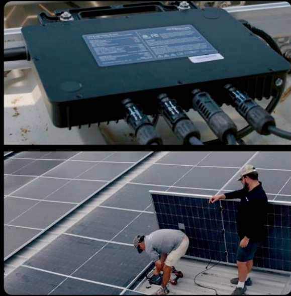
Microinverter Texas, USA Capacity 117kW
