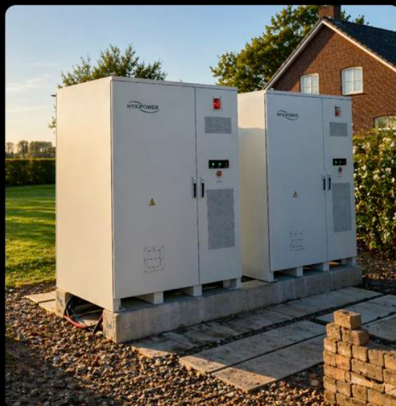
105kW/232kWh C&I ESS Netherlands, Capacity 200kW/430kWh
