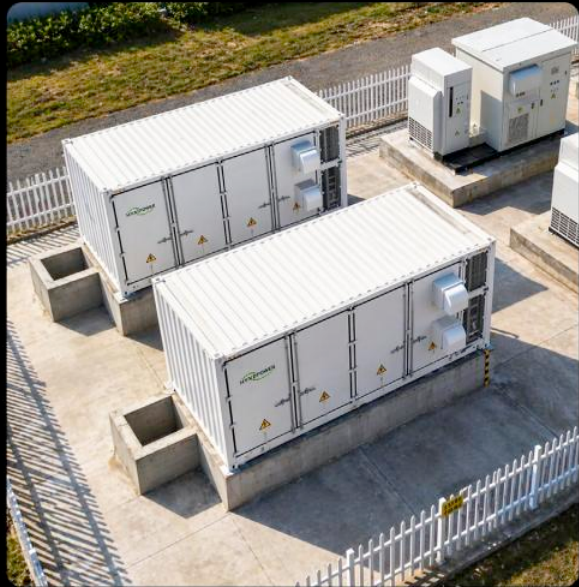
5000kWh Container ESS Zhejiang, China, Capacity 5MW/10MWh
