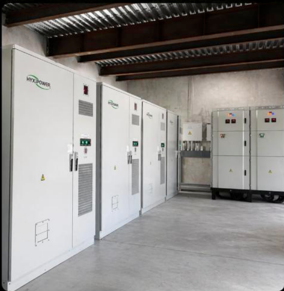
105kW/232kWh C&I ESS Myanmar, Capacity 500kW/1075kWh
