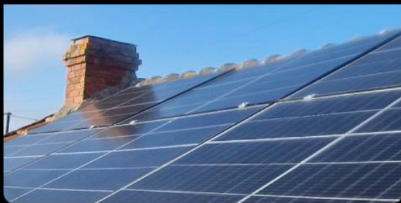
Microinverter Île-de-France, France, Capacity 2.46kW
