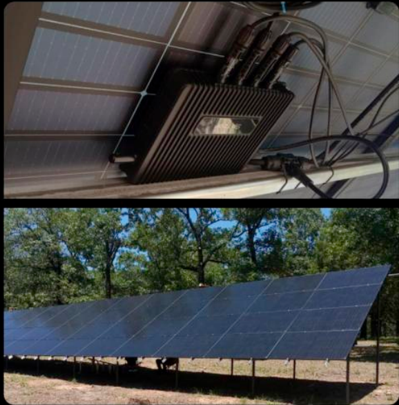
Microinverter Arkansas, USA, Capacity 11.6kW
