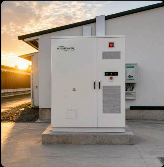
105kW/232kWh C&I ESS Spain, Capacity 100kW/215kWh
