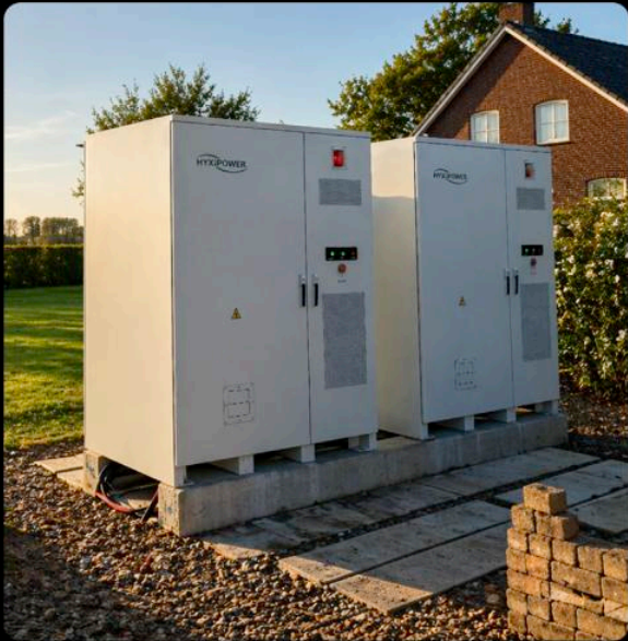
105kW/232kWh C&I ESS Netherlands, Capacity 200kW/430kWh
