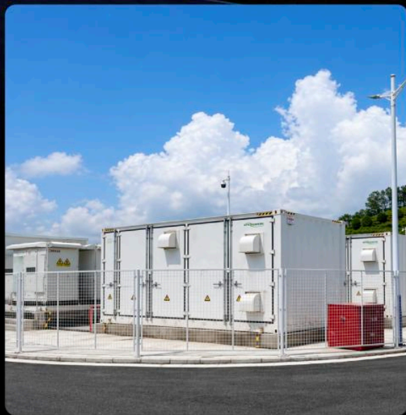
5000kWh Container ESS Zhejiang, China, Capacity 400MWh
