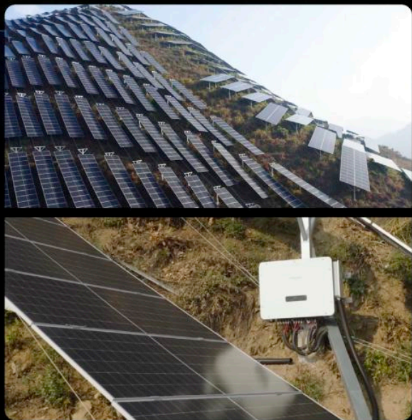
String Inverter Hangzhou, China, Capacity 40MWp
