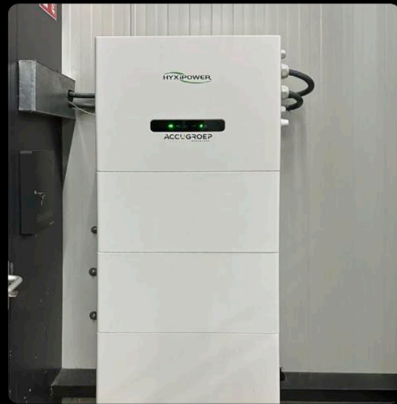
All-in-One ESS Overijssel, Netherlands, Capacity 12kW/20kWh
