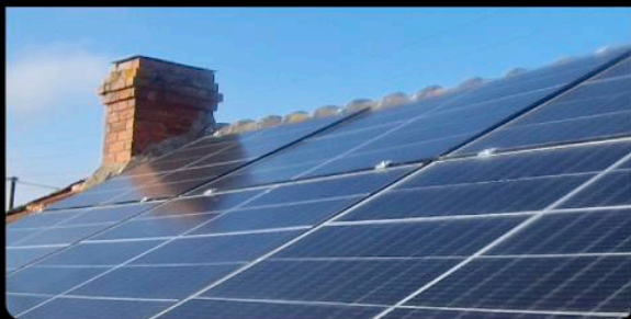
Microinverter Île-de-France, France, Capacity 2.46kW
