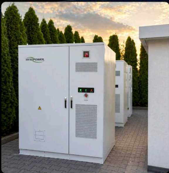
100kW/215kWh C&I ESS Poland, Capacity 200kW/430kWh
