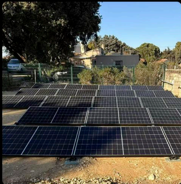
Microinverter Orange, France, Capacity 9kW
