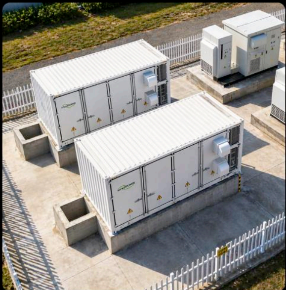
5000kWh Container ESS Zhejiang, China, Capacity 5MW/10MWh
