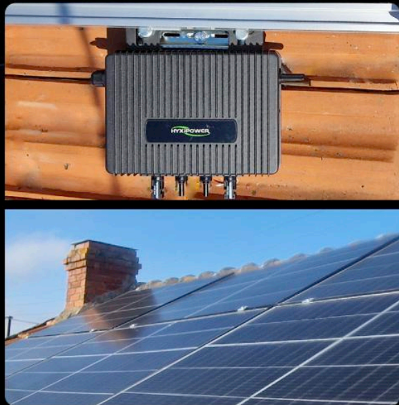
Microinverter Île-de-France, France, Capacity 2.46kW
