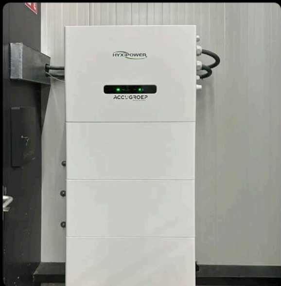
All-in-One ESS Overijssel, Netherlands, Capacity 12kW/20kWh
