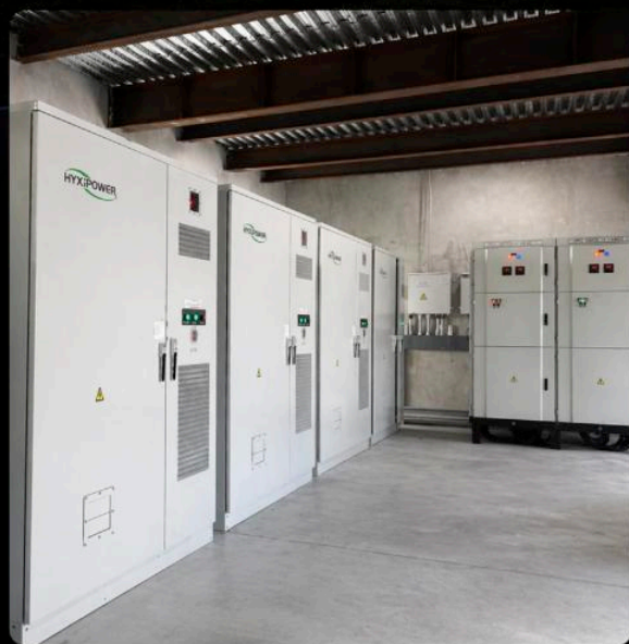
105kW/232kWh C&I ESS Myanmar, Capacity 500kW/1075kWh
