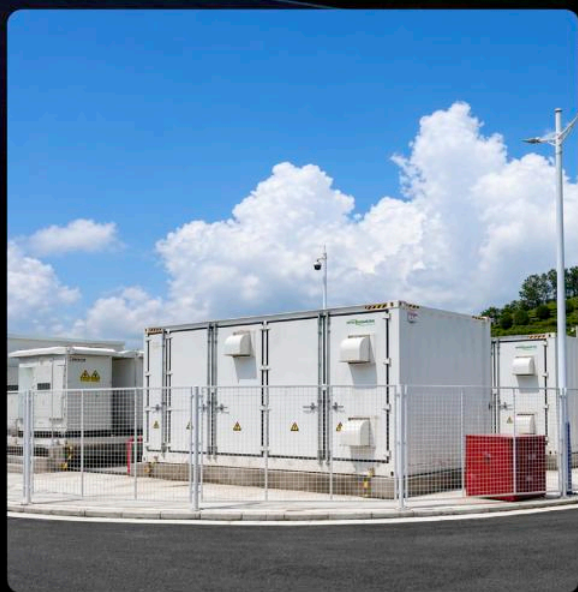
5000kWh Container ESS Zhejiang, China, Capacity 400MW/h
