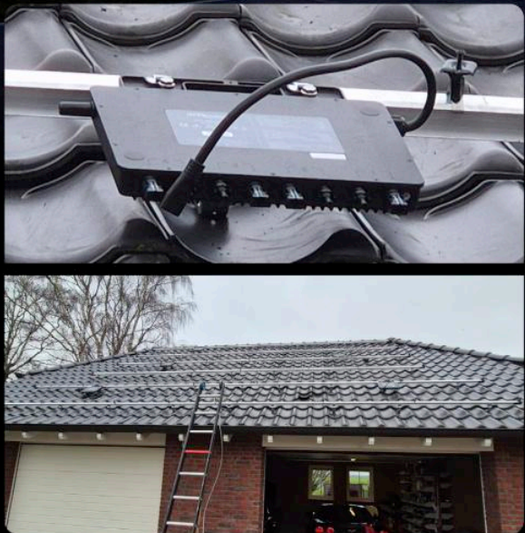
Microinverter Drenthe, Netherlands, Capacity 7.9kW
