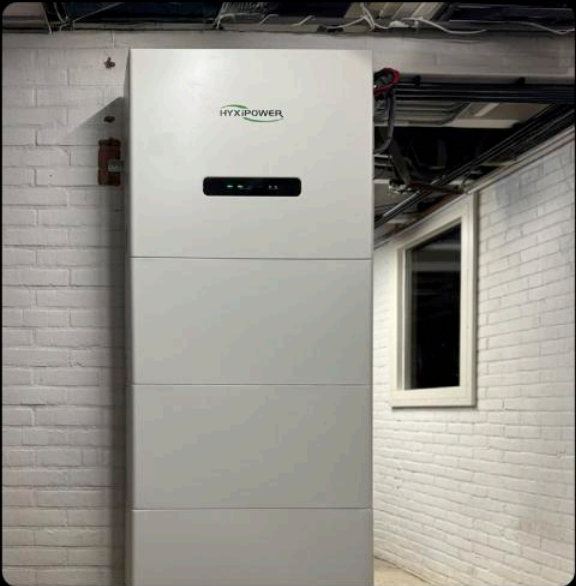
All-in-One ESS Overijssel, Netherlands, Capacity 12kW/20kWh
