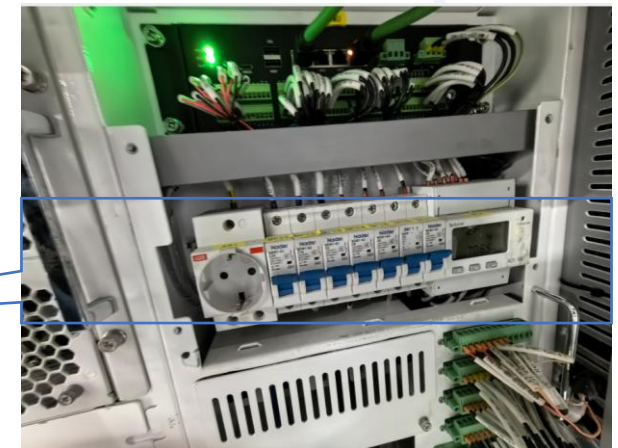
Cabinet power supply breakers
