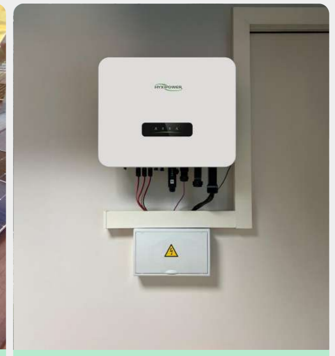
Hybrid Inverter Lleida, Spain Capacity 25kW
