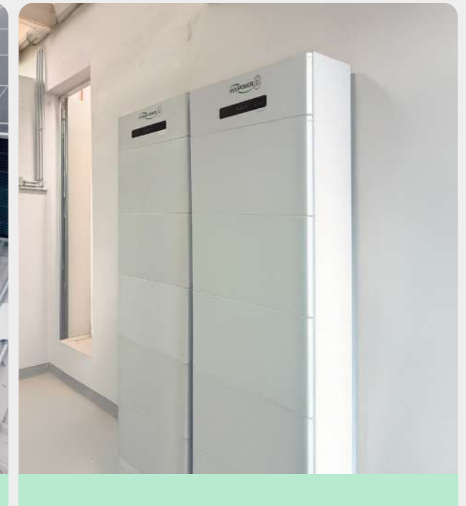
Hybrid Inverter, High Voltage Battery Bad Neuenahr-Ahrweiler, Germany Capacity 50kW/50kWh
