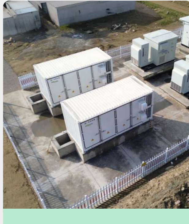
5000kWh Container ESS Zhejiang, China Capacity 5MW/10MWh
