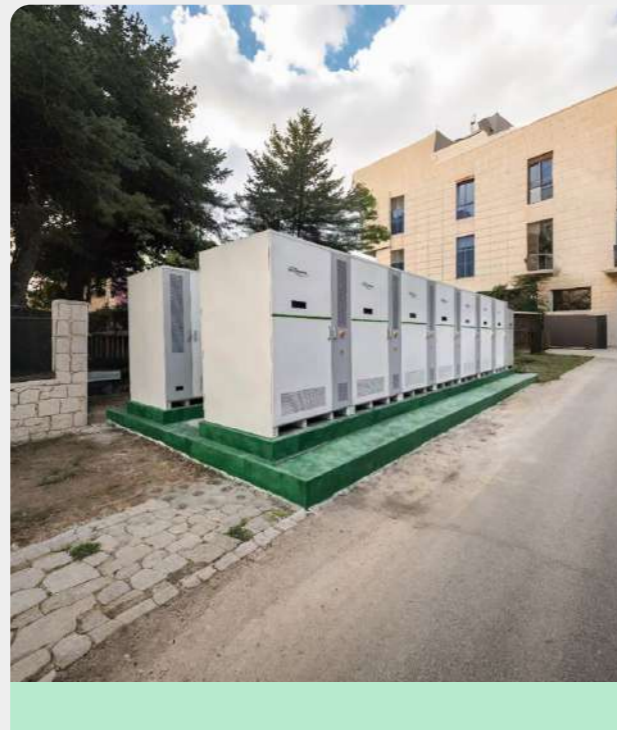
105kW/232kWh Liquid Cooling ESS Guangdong, China Capacity 2.32MW/4.64MWh
