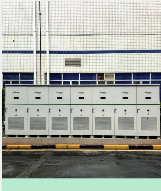
105kW/232kWh Liquid Cooling ESS Guangdong, China Capacity 3.25MW/7.19MWh
