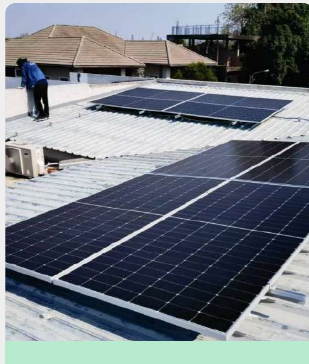
4-in-1 Microinverter Bangkok, Thailand Capacity 5kW
