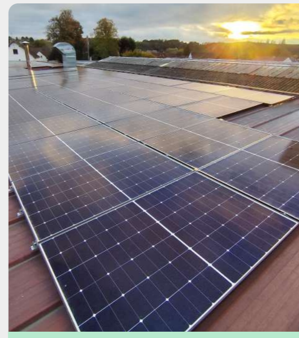
String Inverter Nogent-le-Roi, France Capacity 40kW
