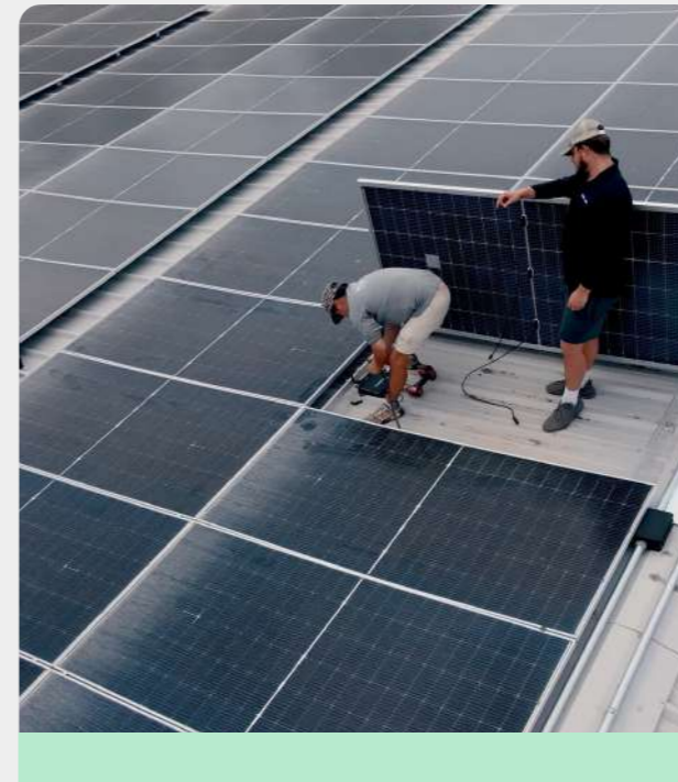
4-in-1 & 2-in-1 Microinverters Nacogdoches, Texas, USA Capacity 117kW
