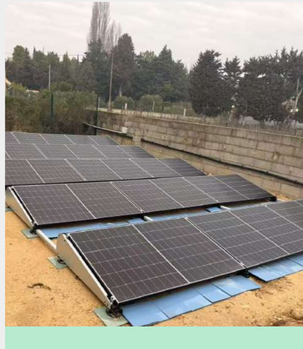
2-in-1 Microinverter Orange, France Capacity 9kW
