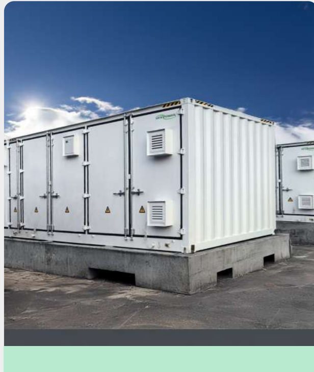
5000kWh Container ESS Zhejiang, China Capacity 400MWh
